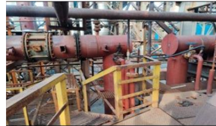
Throttle and U seal ( U seal of existing C.O. gas line used)
